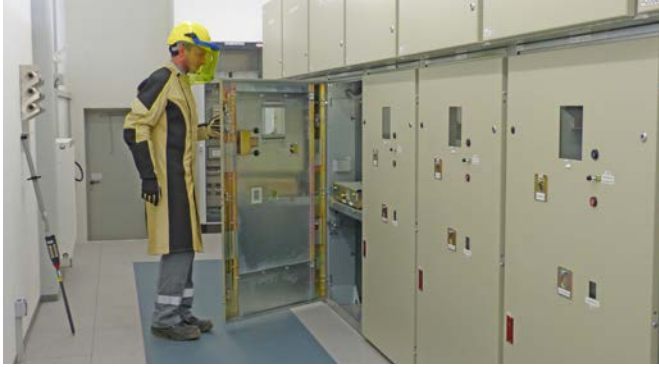
Switch room with insulating mat fitted.
