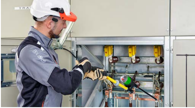
Single-pole PHV I phase comparator used in a switchgear installation.
