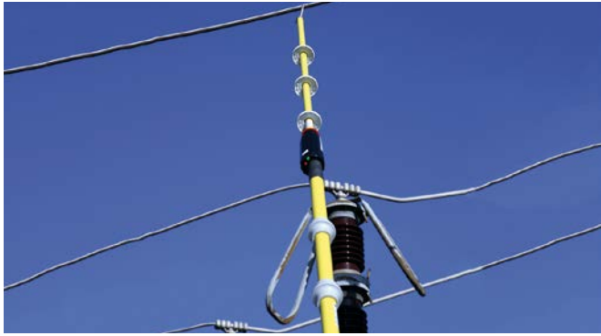
PHE III voltage detector used on a 110 kV outdoor station.
